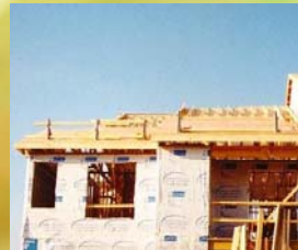
Slide guards with guardrails for sheathing
